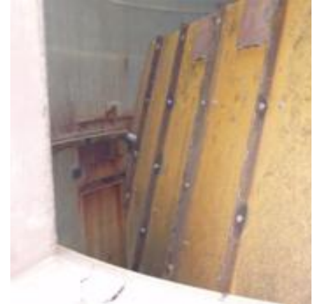
Open Stack Damper
